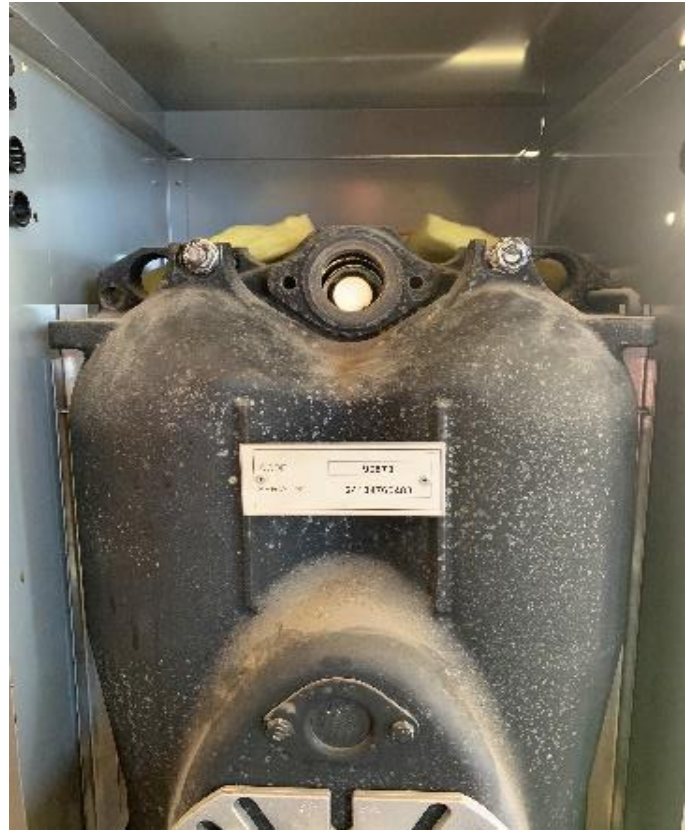
Odyssey boiler with the well removed
