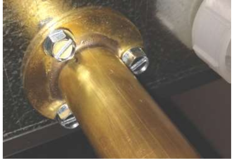
Pressure relief valve connection
