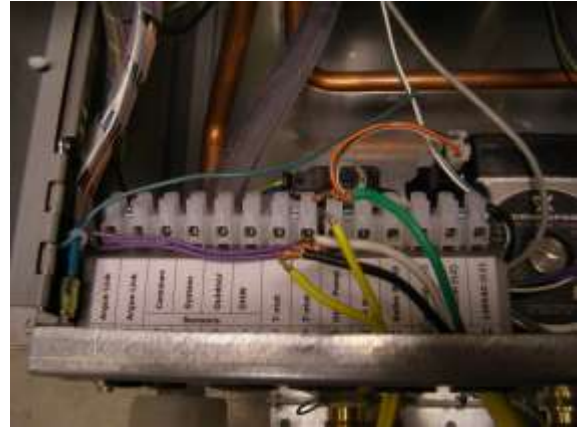
Wiring Terminal Strip
